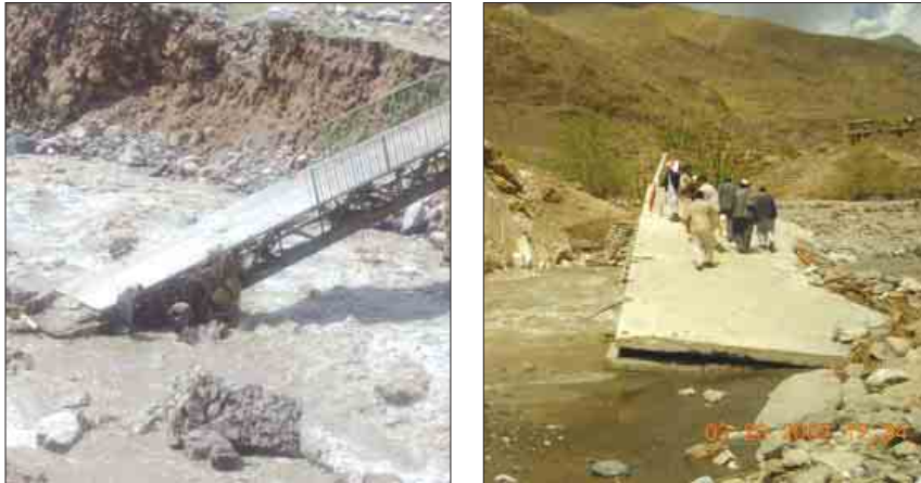
Figure 2c: Collapsed bridges in Kolomai and Salang district in Parwan Province.
