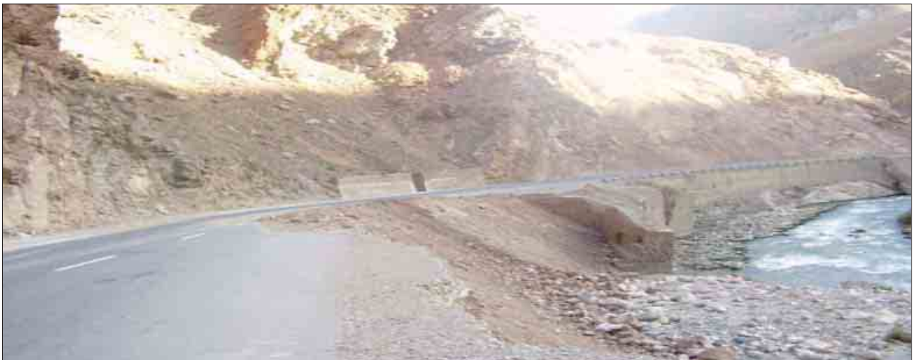
Figure 2a: The highway connecting the north to the capital city, Kabul. The reconstruction of this highway was completed in 2005 but several sections of this road have being severely damaged by flooding after a year due to poor design.
