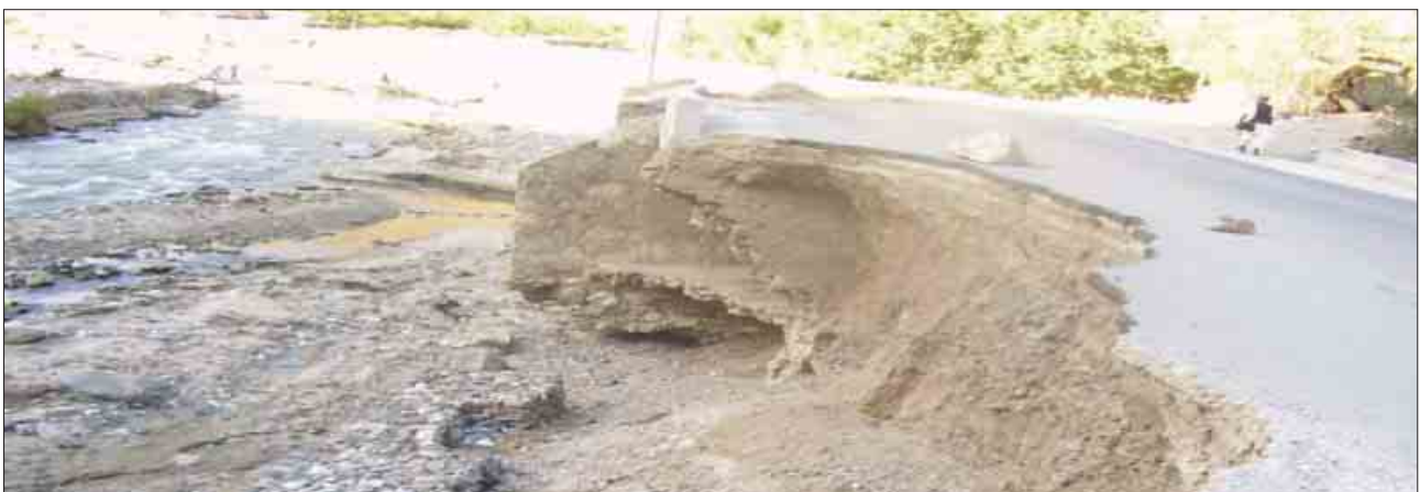
Figure 2b: A section of the highway near Salang damaged by flooding in May 2007.
