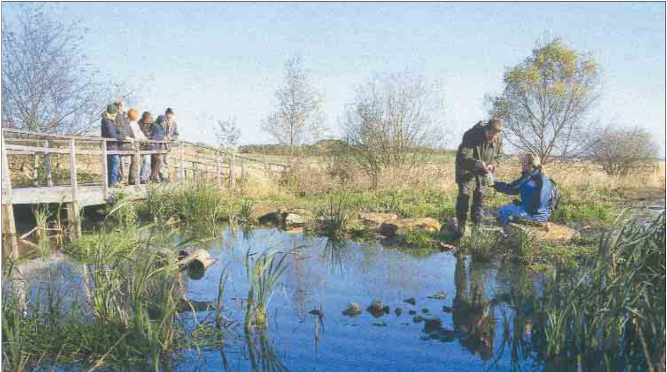
The completed full-scale wetland treatment system at Quaking Houses built by local community volunteers
