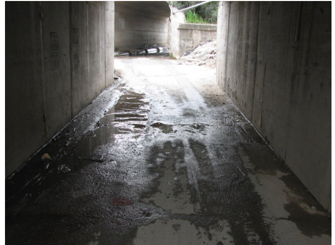
Figure 4 the undercrossing without drainage is unsafe when it rains
