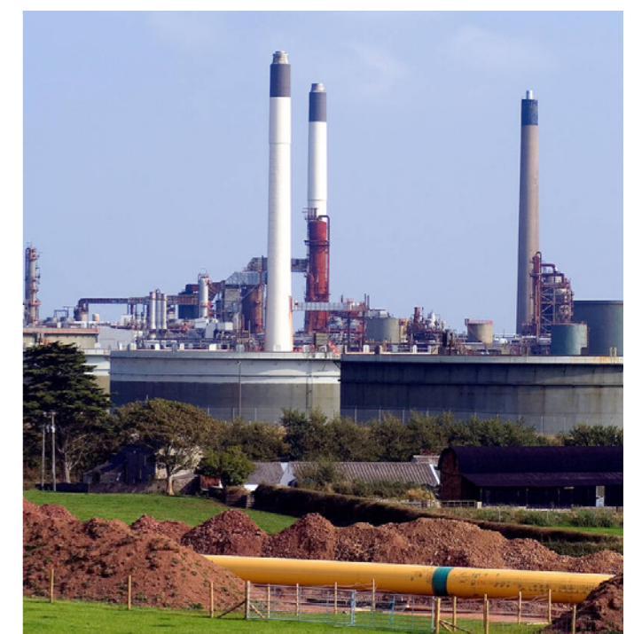
Laying an LNG pipeline running from Milford Haven to England. Photo: Alamy
