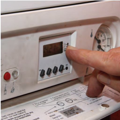
Figure 16: Boiler control panel
