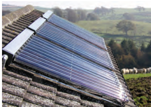
Figure 14: Solar thermal collectors
