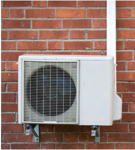
Figure 9: Air-source heat pump – external heat exchanger
