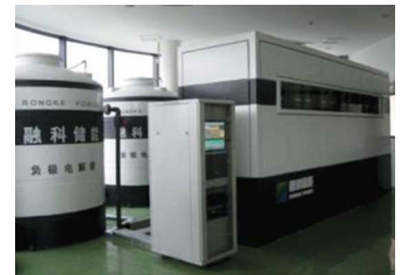
Fig.4 A 60kW/300kWh VRB system in Rongke Power Company R&D building
