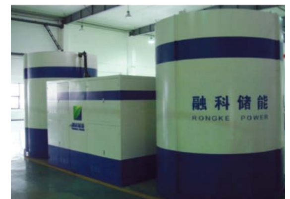
Fig.6 A 80kW/160kWh VRB system for grid connection testing in National Grid of China
