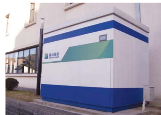
Fig.5 A 3.5kW/54kWh VRB system for telecom station
