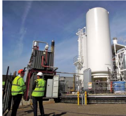
Highview Cryogenic energy storage Demonstrator Plant in Slough, UK
