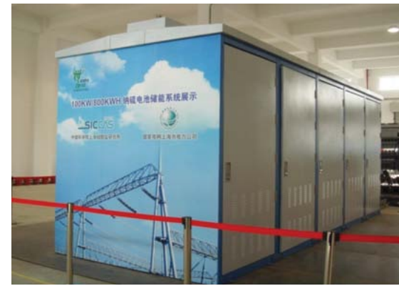
Fig.8 A 100KW/800KWh energy storage system
