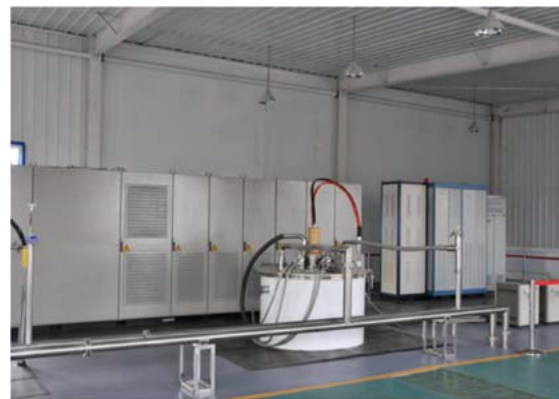
Fig.9 1MJ/0.5MVA, the whole system of SMES
