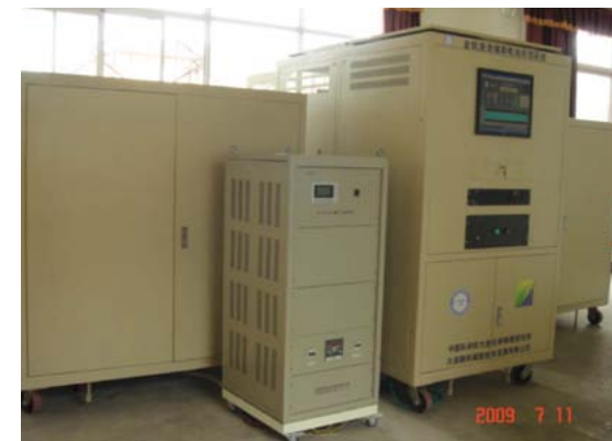
Fig.3 A 5kW/50kWh VRB system for off-grid PV-VRB joint power supply system in Tibet
