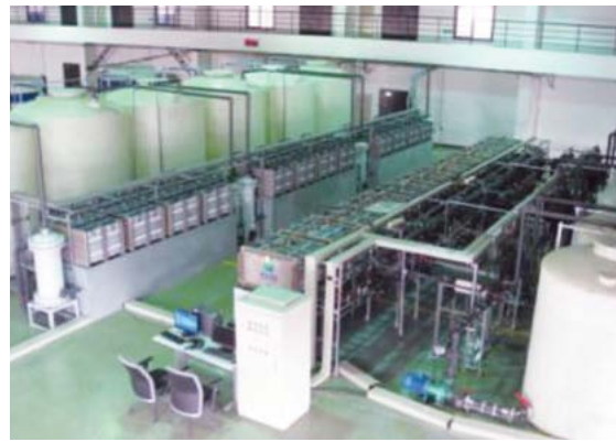
Fig.7 A 520kW/1000kWh VRB testing system
