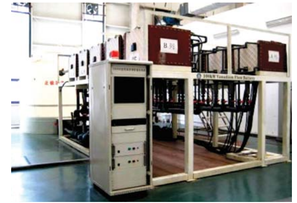
Fig.2 A 100kW/200kWh VRB system for grid connection system
